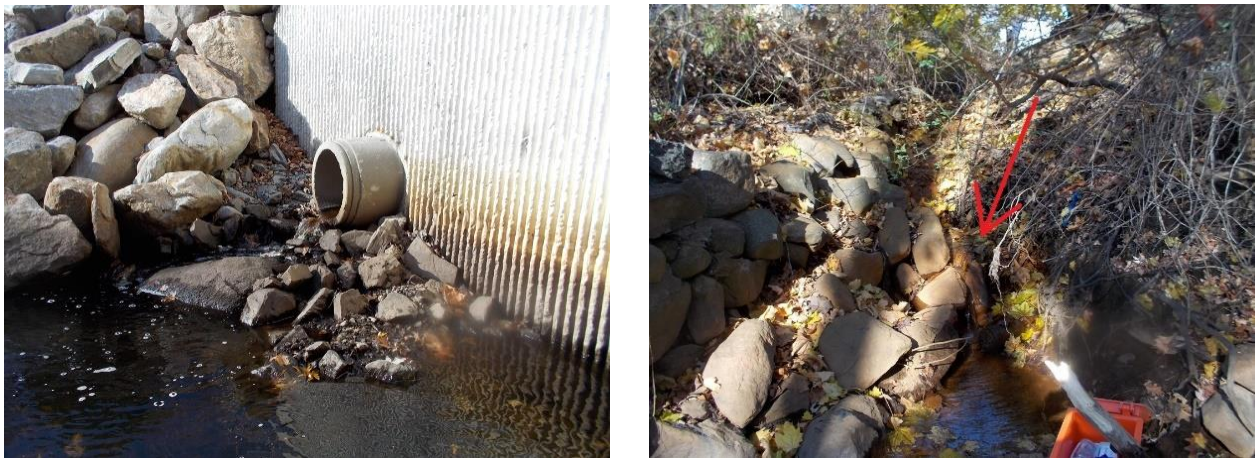
Figure 6: Inflows with high detergent levels (mile 8.15 on left next to Florida Rd. bridge; mile 8.10 on right 200 ft. downstream of Florida Rd. bridge).
